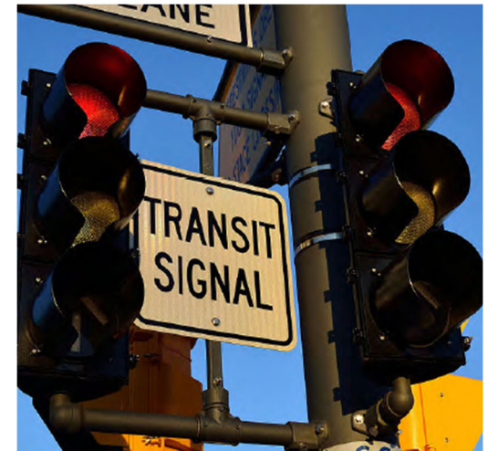
Figure 4.3.13 | Example of TSP signalization at an intersection.
