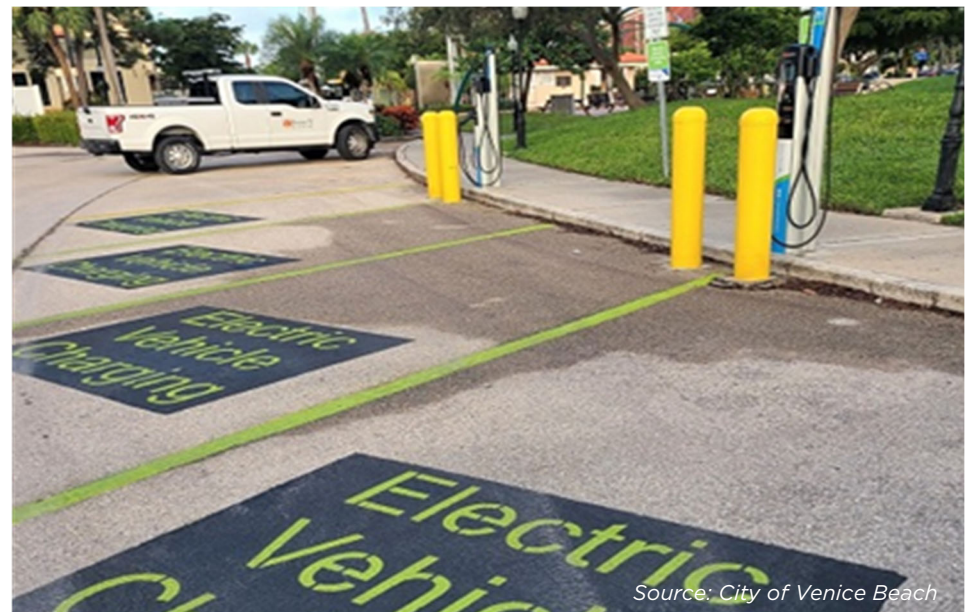
Figure 3.9.4 | EV charging stations in Venice Beach, Florida.
