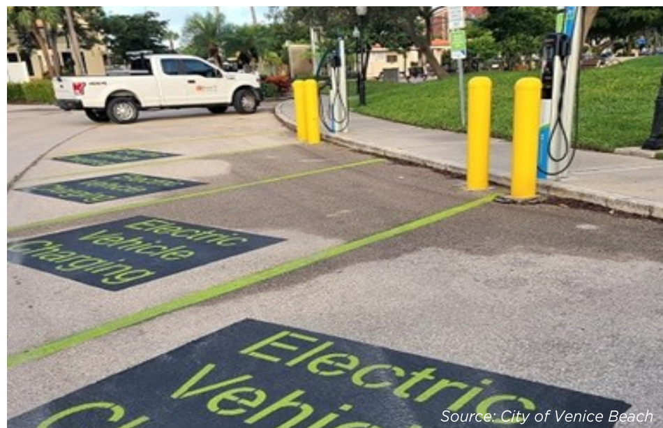
Figure 3.9.4 | EV charging stations in Venice Beach, Florida.
