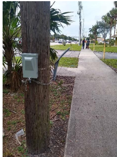
Infrared sensor in closed enclosure box
