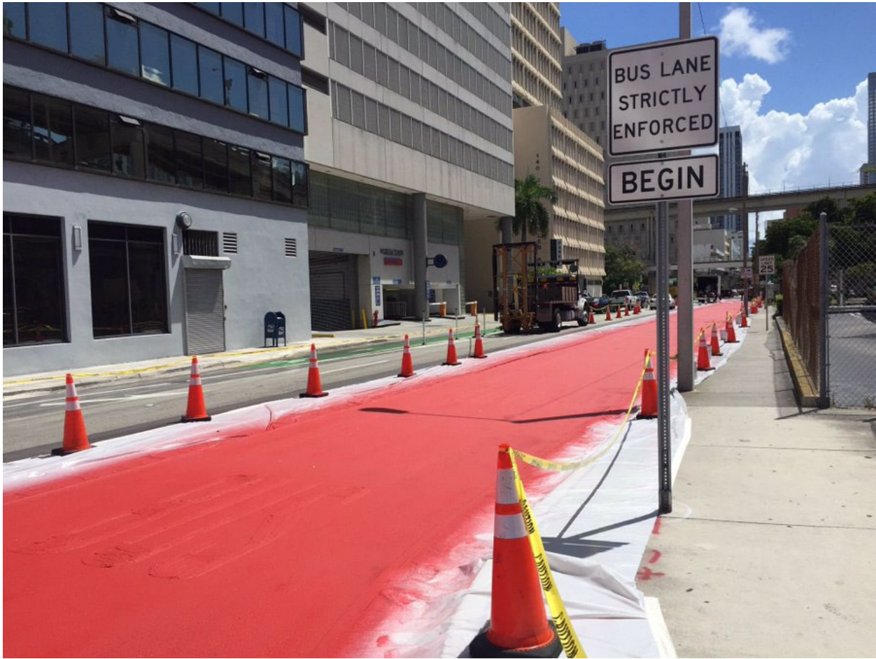
Figure 21: Construction of the SE 1st St Bus Only Lanes in 2017 (Photo: Stephanie Cornejo)
