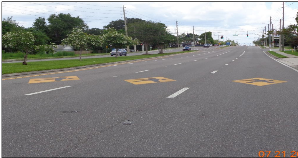
Figure 5.2-3. PEDESTRIAN CROSSING WARNING Sign (W11-2) Pavement Marking
