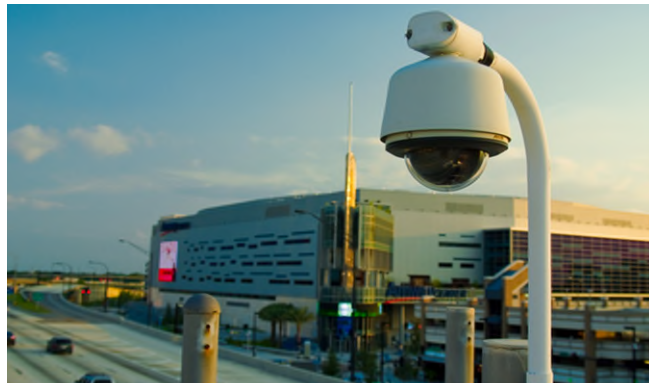
Figure 6: CCTV Camera on I-4 in Orlando
