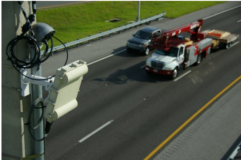
Figure 8: Microwave vehicle detection system
