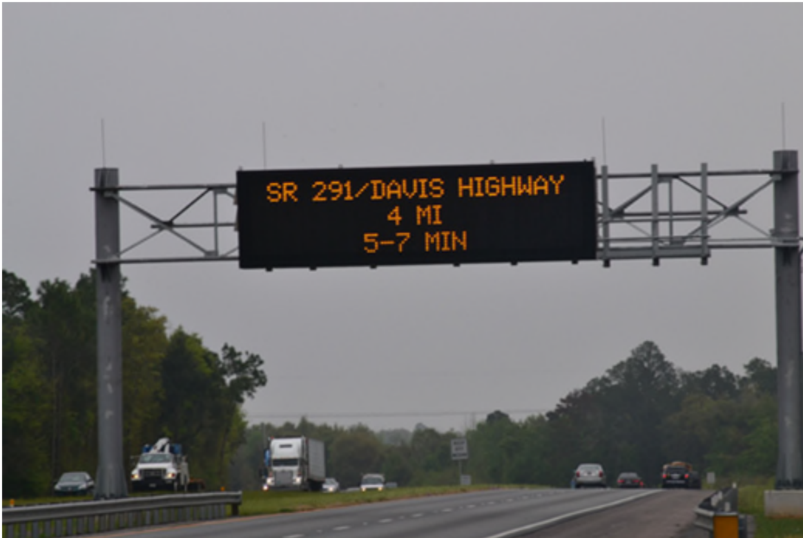
Figure 13: Dynamic Message Sign in Pensacola, Florida
