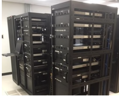
Figure 2: The District One RTMC's Server Room
