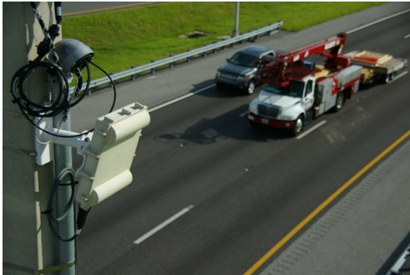
Figure 8: Microwave vehicle detection system
