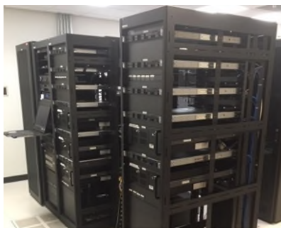
Figure 2: The District One RTMC's Server Room
