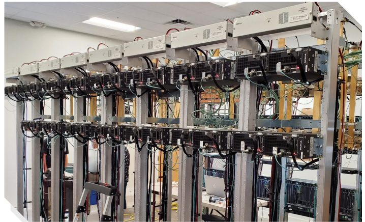
Figure 3 - Microwave Radios Under Test at Staging Facilities
