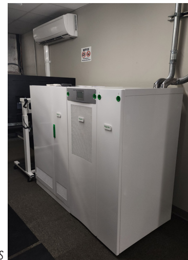
New TMC building UPS
