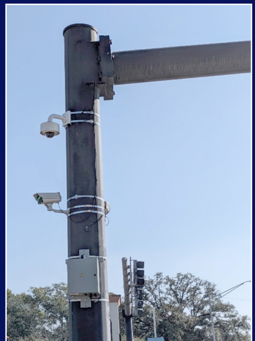
Two images above: US 17 signal mast arm used for technology evaluation
