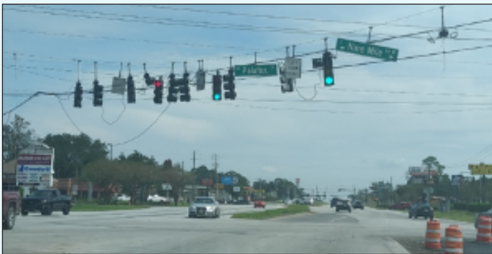
Signal damage from Hurricane Sally
