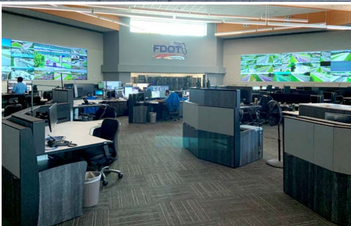
Video walls and operator stations inside of the RTMC command center to help ensure safe and efficient traffic operations.
