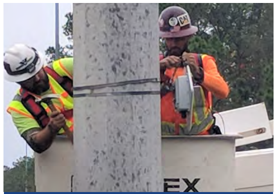
Installing wireless radios on a CCTV pole in Midway to communicate with the ITS Communications Trailer.
