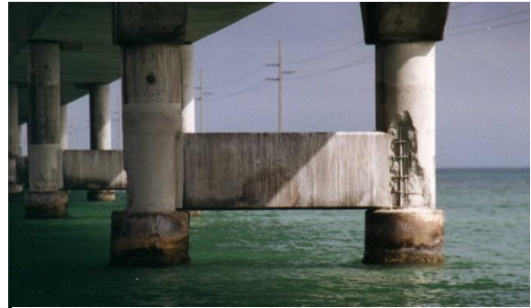
Figure 1: An example of corrosion damage caused by the diffusion of saltwater chlorides into concrete.
