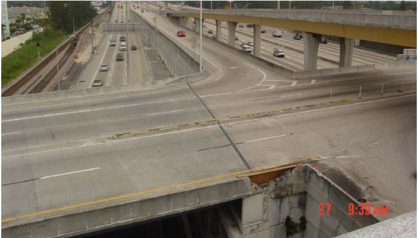
Roadway Conditions Prior to Improvement (Gilbert Soles, FDOT District 4)
