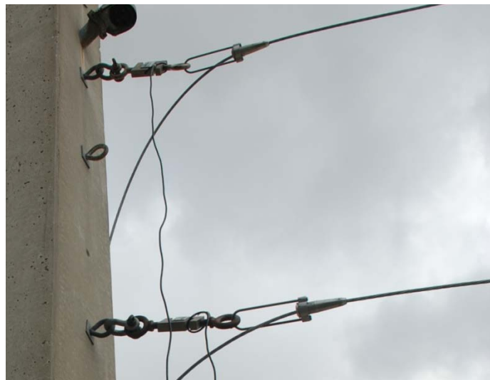
Figure 3-8. Load cells installed in line with catenary and messenger cables (Photo courtesy of author)
