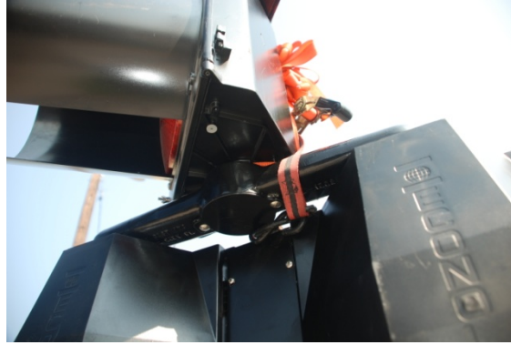
Figure 6-1. Failure of the joint between the top signal head and two-way bracket (Test 22) (Photo courtesy of author)
