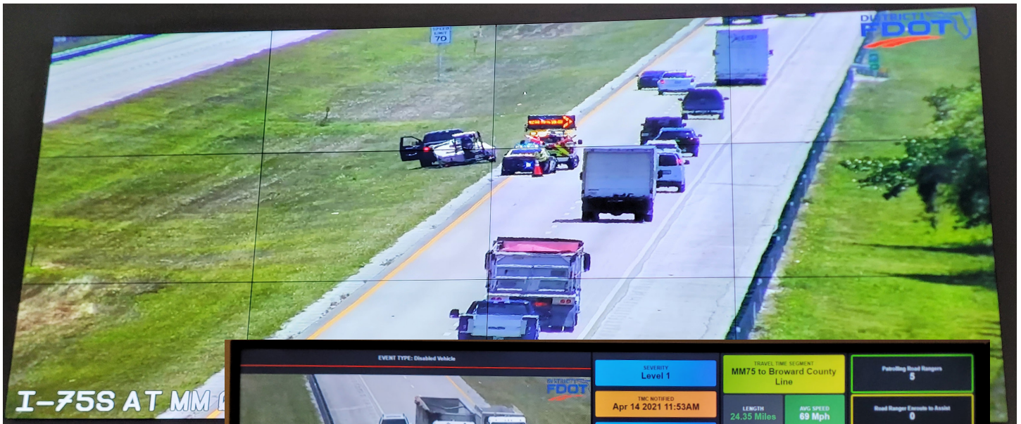
TMC monitoring and response is made more effective with combined video and dashboard displays.
