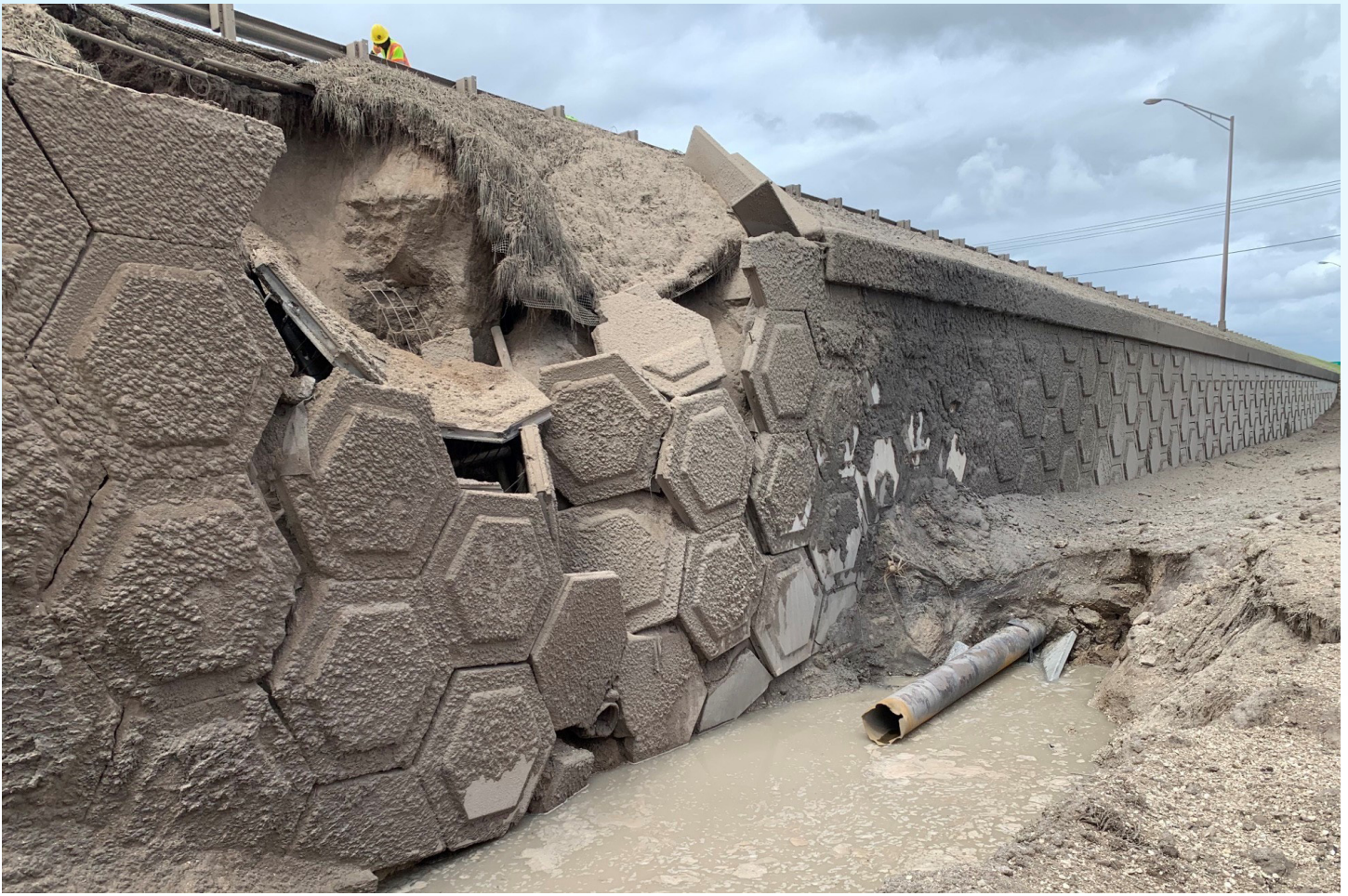
Turnpike retaining wall damage after the gas line eruption.
