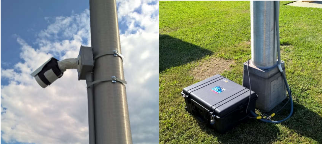
Figure 22. Installed camera, PVC conduit, and Pelican case
