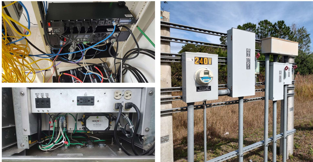
Figure 3-12: Example power infrastructure components including in-cabinet equipment (left) and infrastructure (right)
