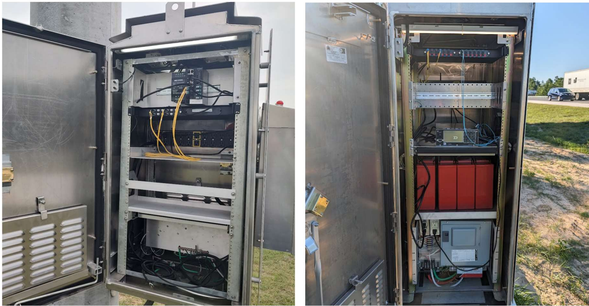
Figure 3-16: Examples of Intelligent Transportation Systems cabinet assembly interiors
