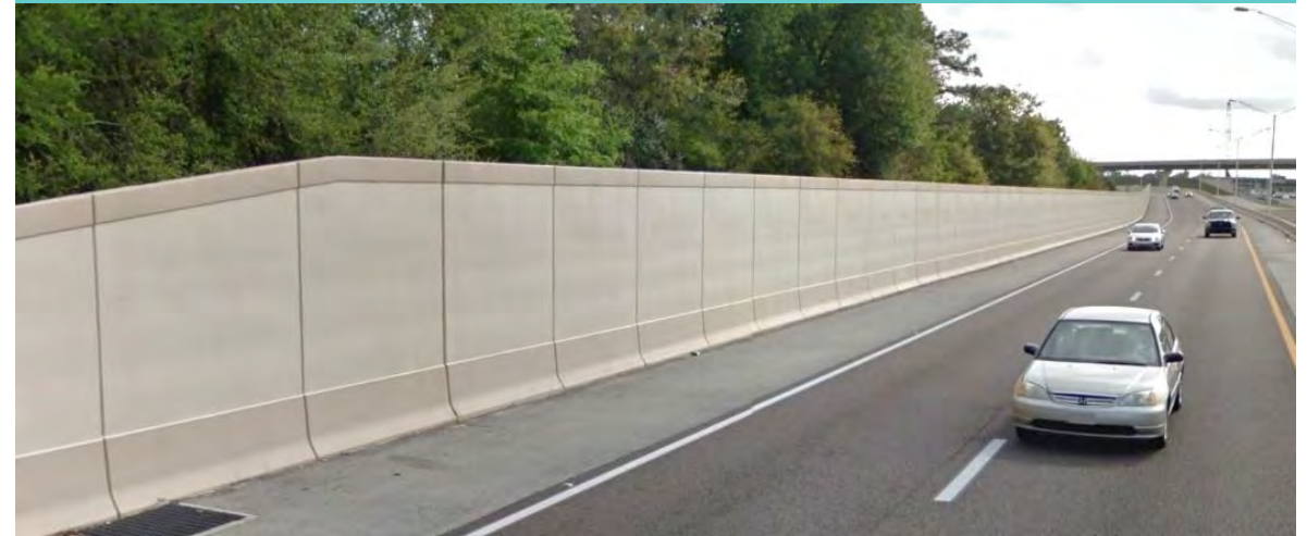
Example shoulder-mounted noise wall
