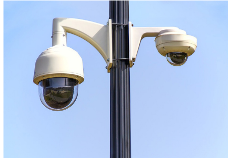
High definition closed-circuit television (CCTV) cameras
