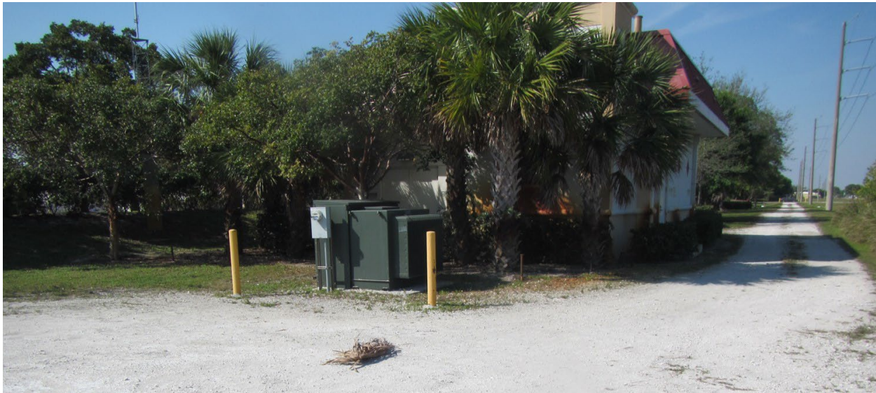
Figure 2.16.2: Existing Pump House
