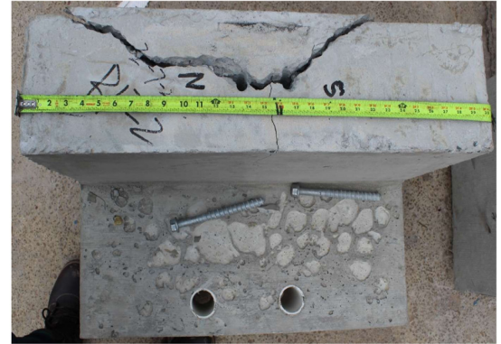
The concrete parapet mockup specimen after breakout of two 5/8-in dia. galvanized screw anchors.
