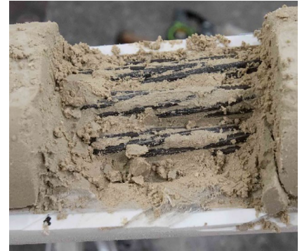
Removing the top of the PVC duct and chiseling away the soft grout exposes the steel strands of a post-tensioning tendon.
