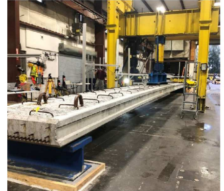
Figure 1. Slab with higher camber than expected.
