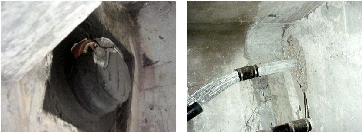
Figure 1-1: Tendon failure on the Mid-Bay Bridge
