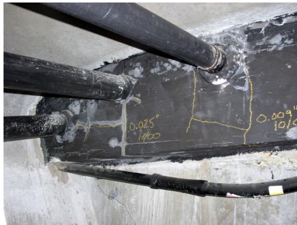
Figure 1-2: Pourback cracking on the Sunshine Skyway Bridge
