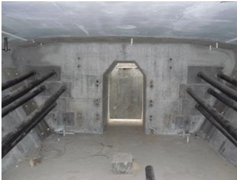
Figure 3-1: Typical concrete dead-end segment. Notice the multiple anchorage points spread throughout the entire segment cross-section.
