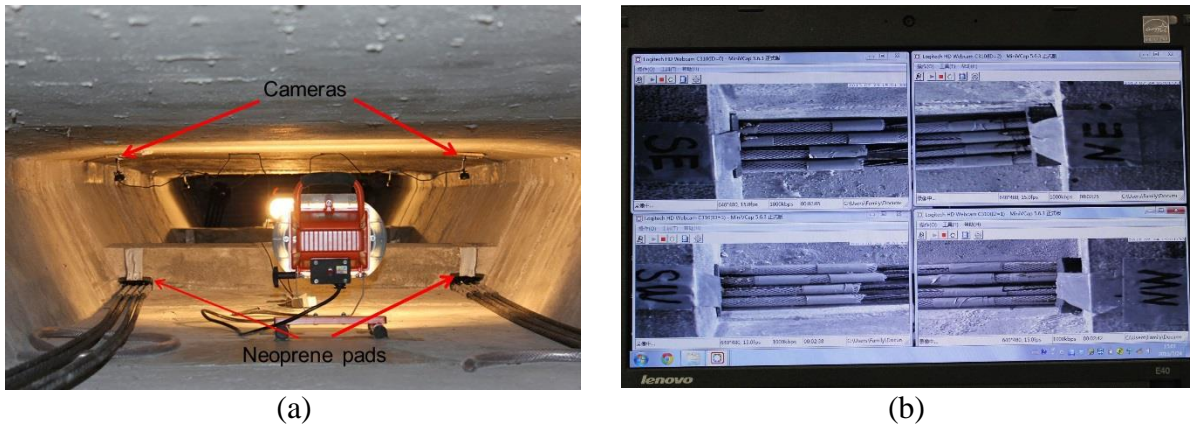
Figure 2.9 Condition-Monitoring of Tendons: (a) Camera inside the Bridge Mode, and (b) Image of Tendons during Tensioning
