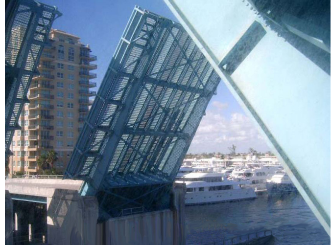
Sunrise Boulevard Bridge in Ft. Lauderdale, shown with its movable leaves in raised position.
