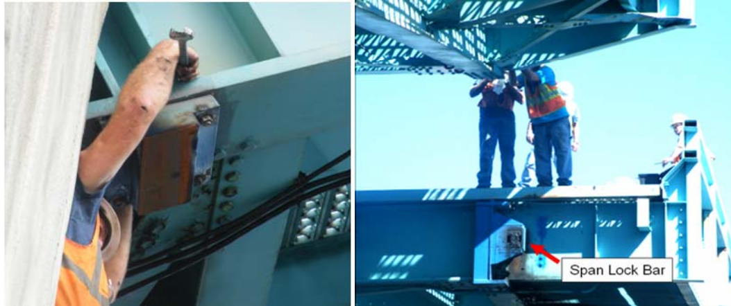
Figure 2: Damage tests (structural): removal of the live load shoe shims (left) and removal of the span lock shims (right)
