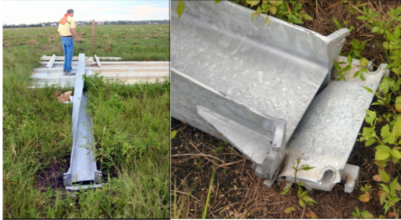
Figure 1-1. Failure of sign structure with slip-base connection under hurricane wind loading
