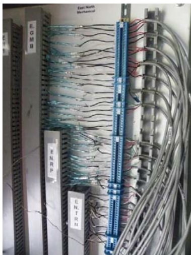
Figure 36: Cable Entries to DIN Rail on Side Junction Box Panel
