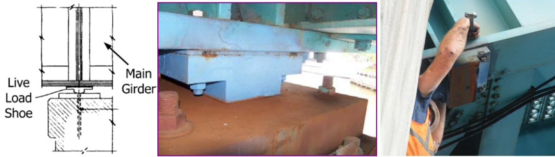
Figure 126: Live Load Shoe (LLS) and the Shim Removal Operation by FDOT Contractors (sketch adapted from Christa McAuliffe Bridge construction plans)
