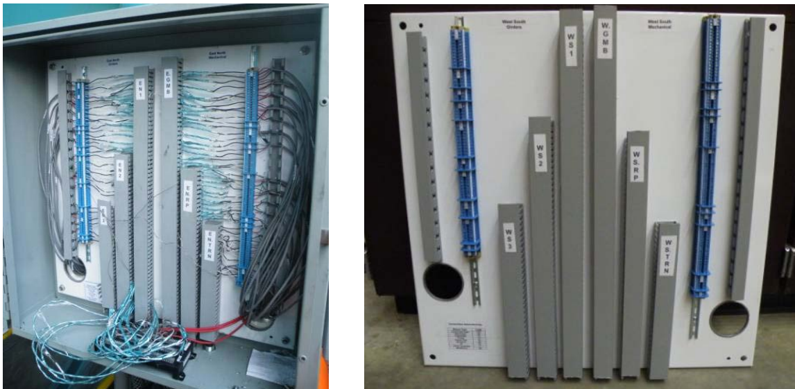
Figure 35: Interior View of Side Junction Box (Left) and Lab Prepared Junction Box Panel (Right)
