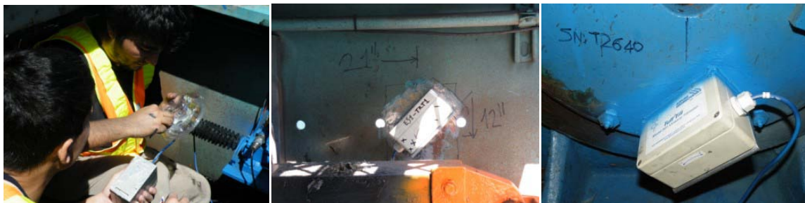
Figure 55: Tiltmeter Installation at the Span Lock Room
