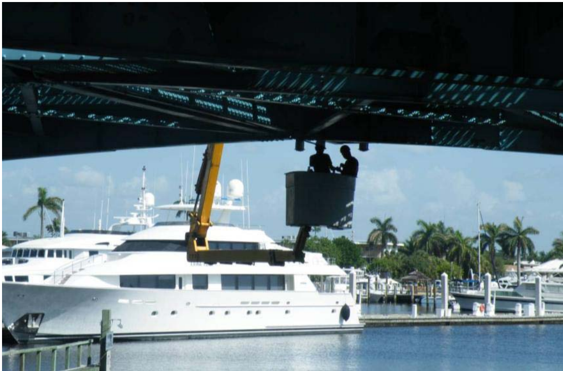
Figure 50: Sensor Installation Under the Bridge
