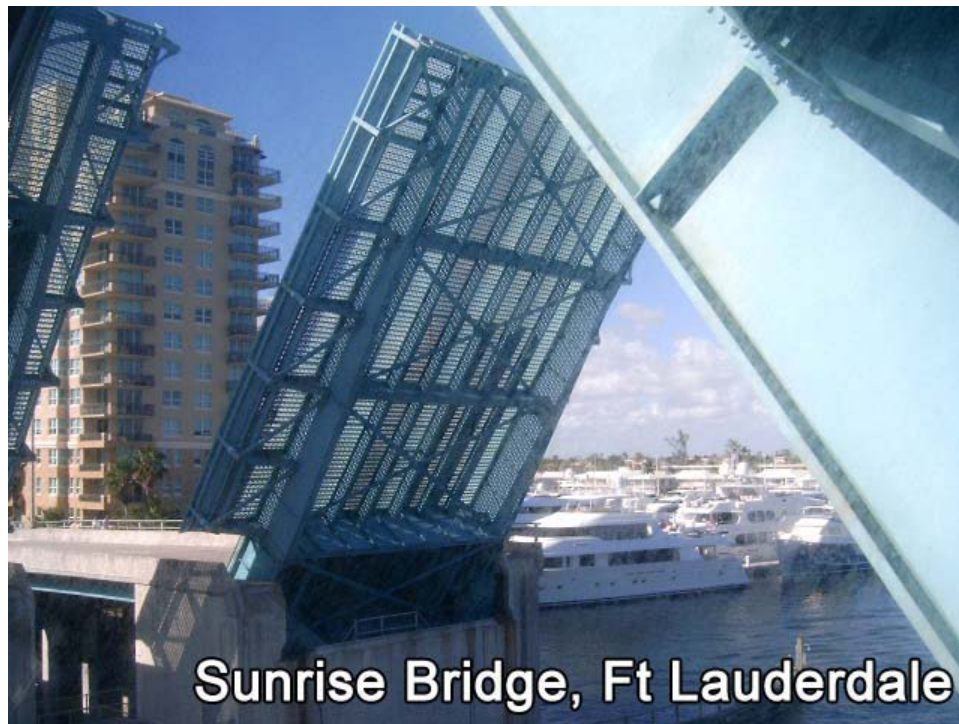
Figure 10: Main Girders in Open Position
