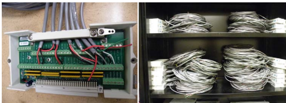
Figure 37: Lab Prepared NI Terminal Block and Completed NI Terminal Blocks Ready for Field Installation
