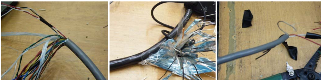
Figure 47: Grey Cable (Left), Black Cable (Center), Sensor Wire (Right)
