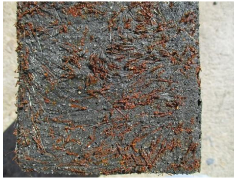
Photo 4.7. Rust on exposed steel fibers.
