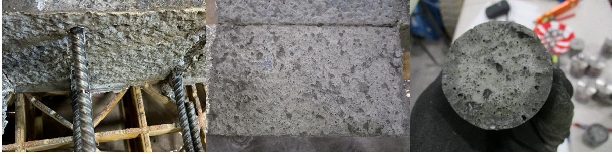
Photo 5.2. Pores at surface of deficient interface concrete.
