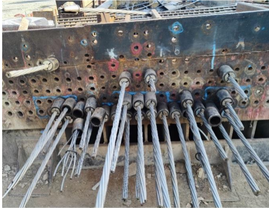
Figure 3-30. Location of the ruptured strands at End 8
