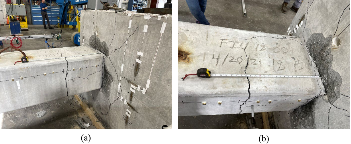
Figure 5.89: Photographs of the failure of SP-03.
