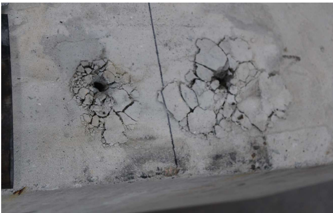
Figure A-122: G-G-310 specimen concrete after breakout
