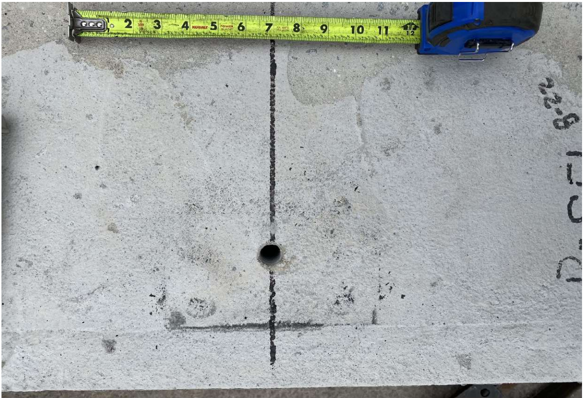
Figure A-24: P-SE1c-4 specimen concrete after cyclic loading
