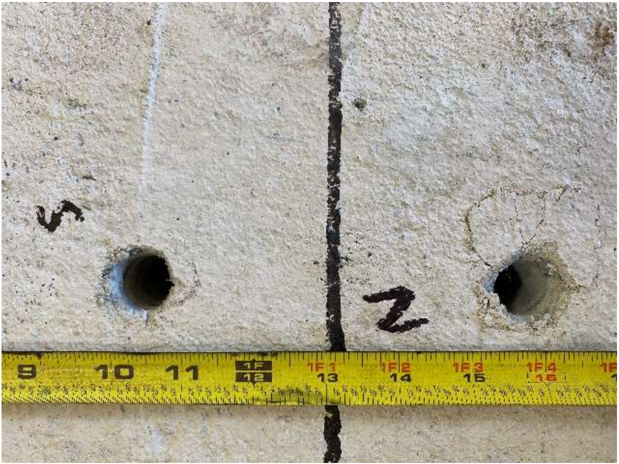
Figure A-49: G-SS-2 specimen concrete after loading
