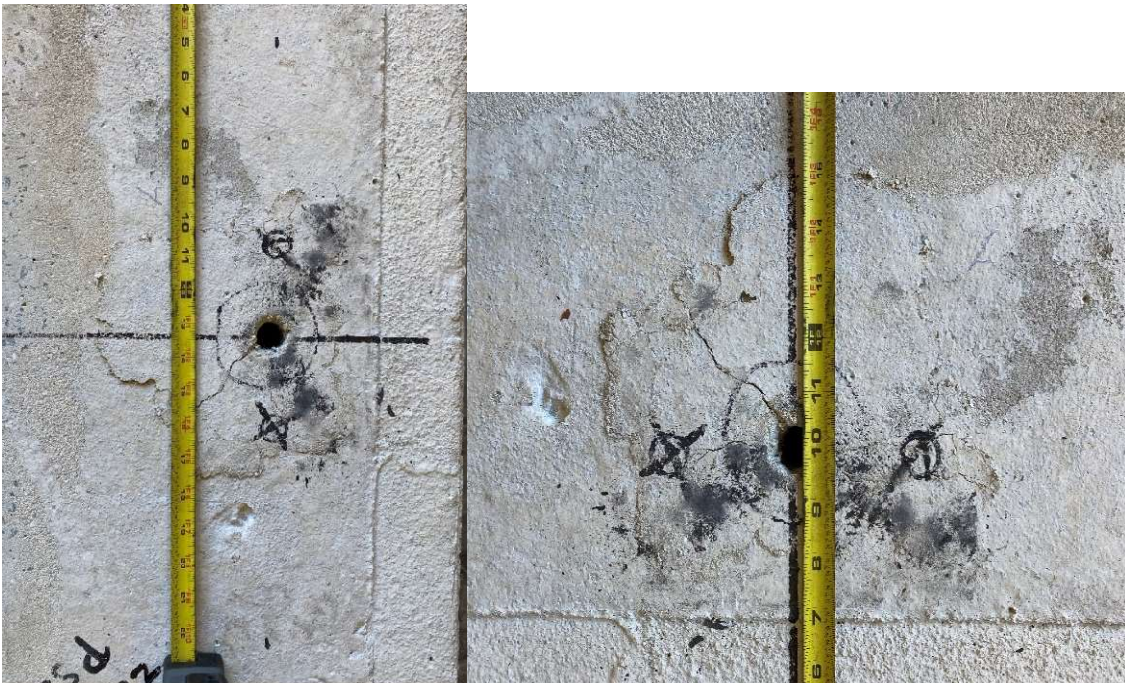
Figure A-8: P-SE1-2 specimen concrete after loading
