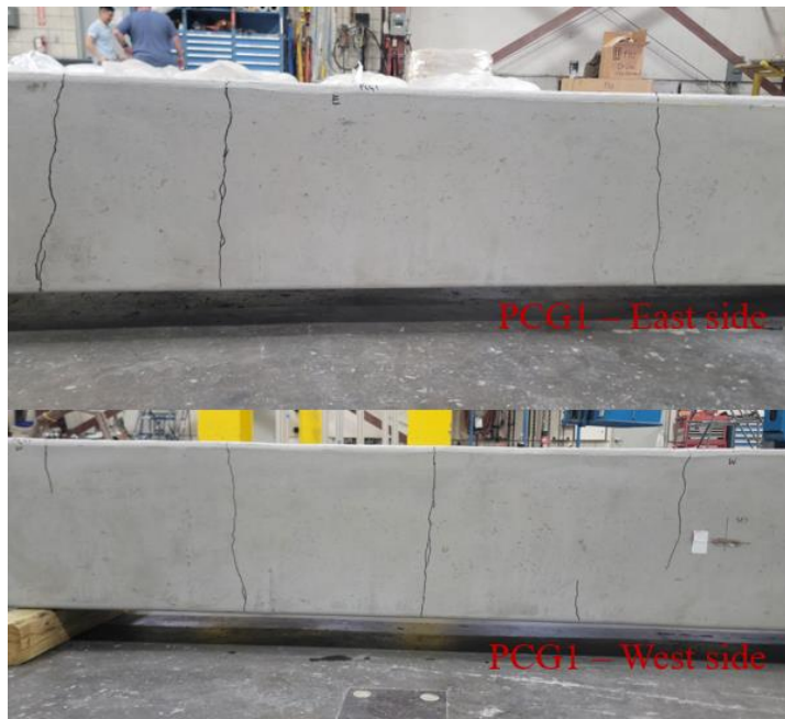
Figure 6.41: Crack pattern after final impact for PCG1
