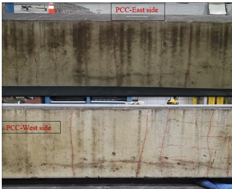
Figure 4.38: Crack pattern after final impact for PCC
