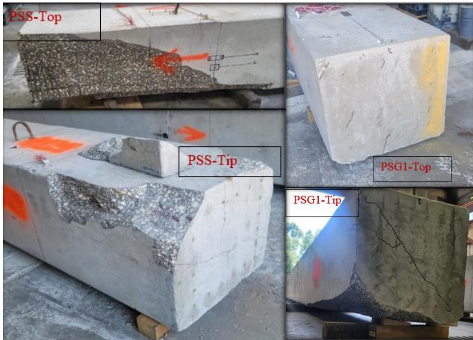
Figure 4.35: Failure at top and tip after final impact for PSS and PSG1
