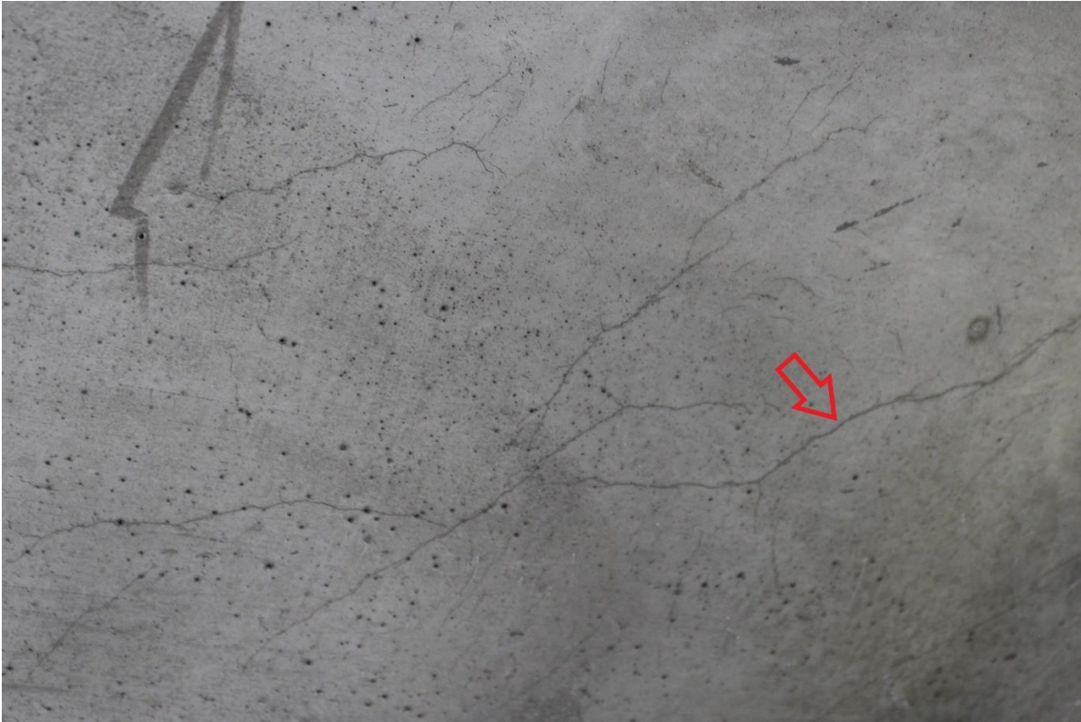
Figure 20; Shrinkage cracking in Slab 2, Row 3 before testing
