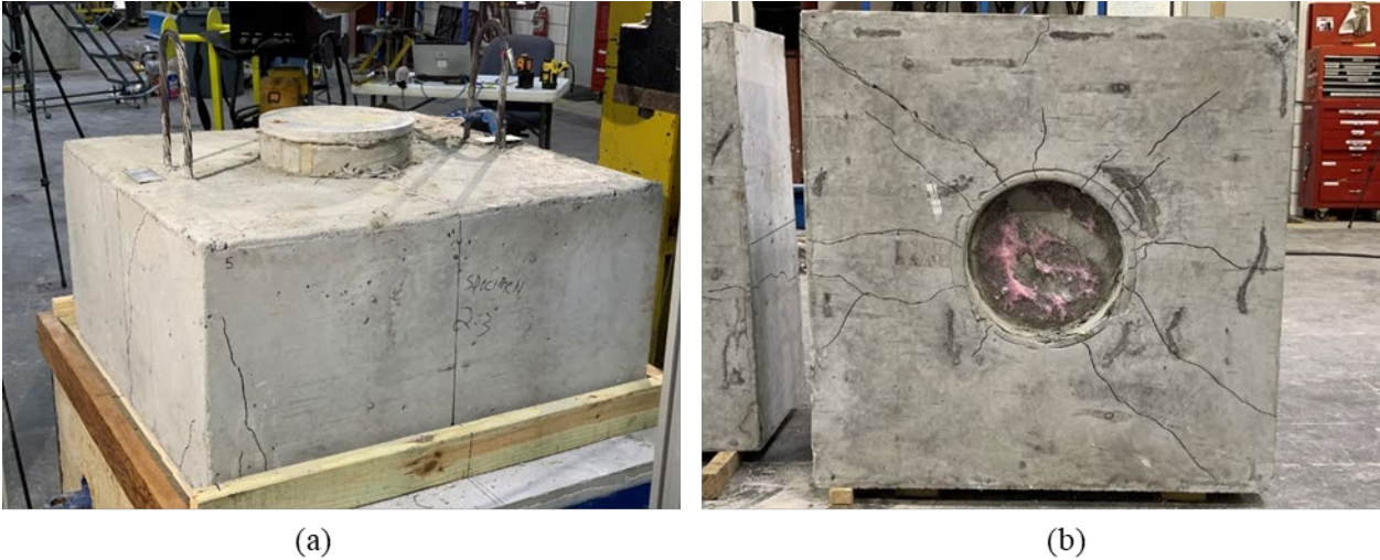
Figure A.38: Cracking on (a) cap and (b) bottom of the Specimen S2-3
