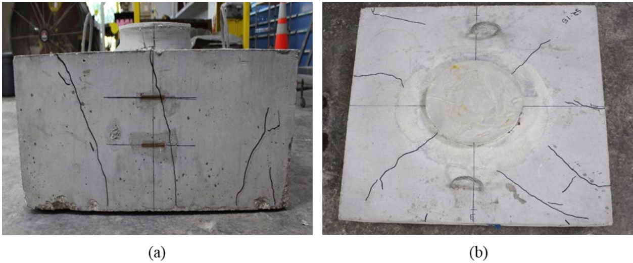
Figure A.118: Cracking on the (a) north side and (b) top of the cap
