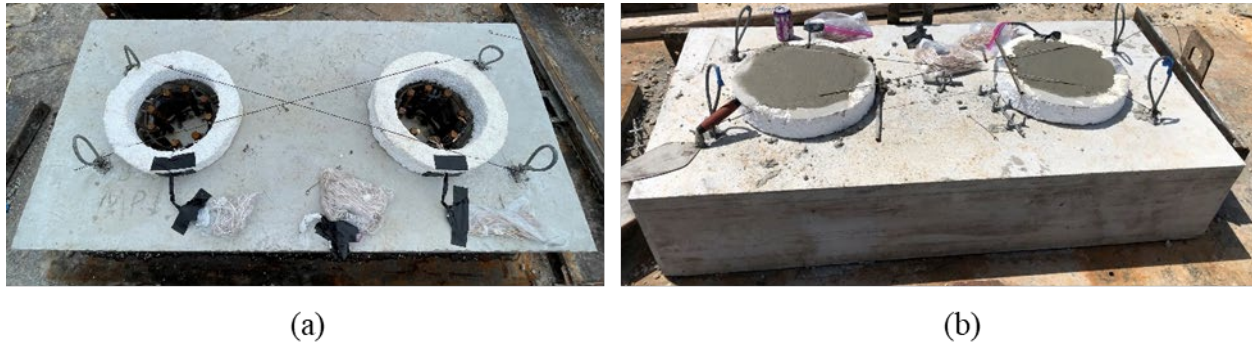
Figure 4.12: Casting of the plug: (a) 3-inch form and reinforcement was placed and (b) concrete was cast.
