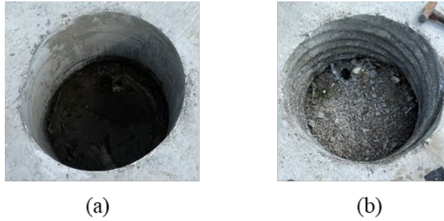
Figure 4.2: Surface finish after removal of pipe with (a) Sonotube and (b) corrugated pipe.
