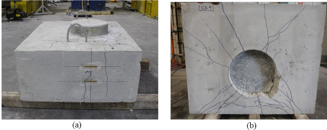
Figure A.197: Cracking on (a) cap and (b) bottom of Specimen S3-9
