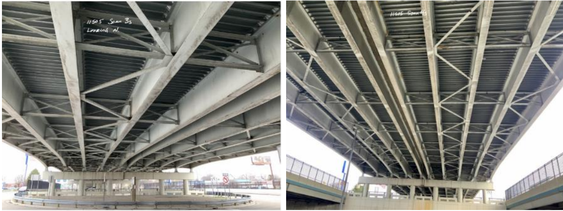
Figure 5-15. Photos from inspection report (Left: Span 3s, right: Span 4s)
