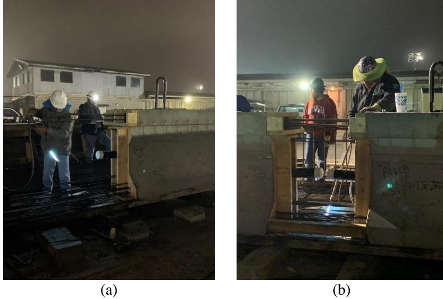
Figure 5.17 Detensioning of SS specimens at (a) east end of prestressing bed and (b) between specimens SS-2 and SS-3
