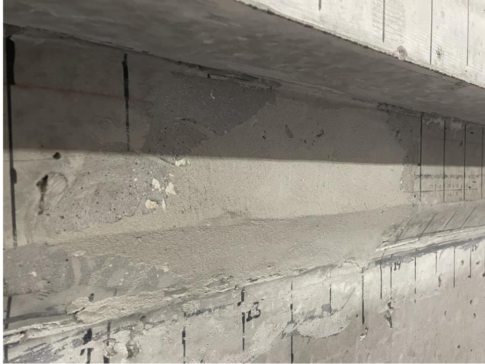
Figure 7.12 Top flange repair on beam specimen NB-3
