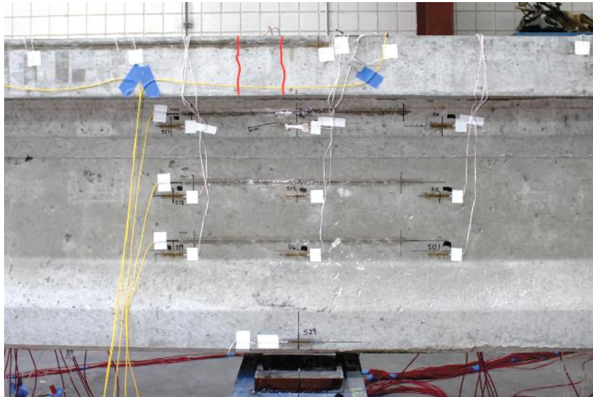
Figure E.37 Specimen NB-3: first observed cracks (marked in red) at P = 102 kip on east side
