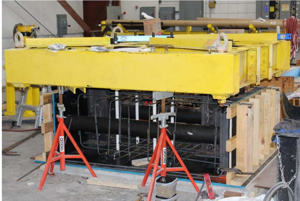
Figure 4.13 Steel hanger frame suspended above the concrete block formwork with embedded steel components correctly positioned
