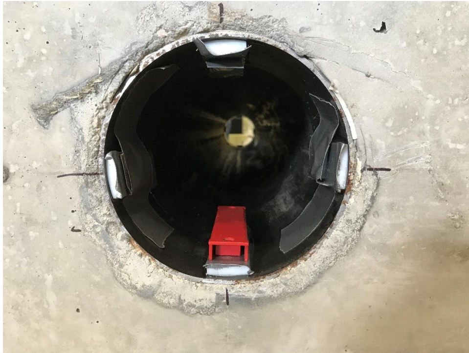
Figure 4.18 Teflon strips positioned within the steel guide tubes with magnets to hold them in place while the adhesive sets
