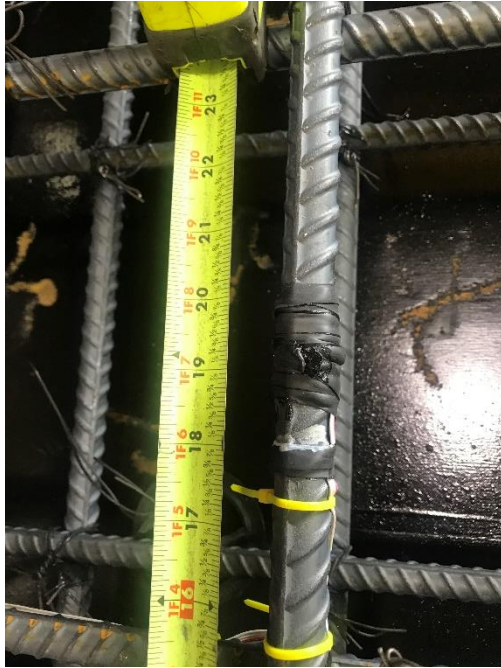
Figure 5.31 Strain gage attached to deck reinforcing bar and protected with waterproof tape
