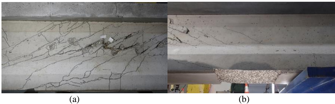
Figure 4-48 Concrete spalling at, (a) web and (b) bottom flange at near support.
