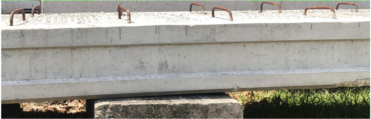
Figure 11 Cracks Noted at the Support
