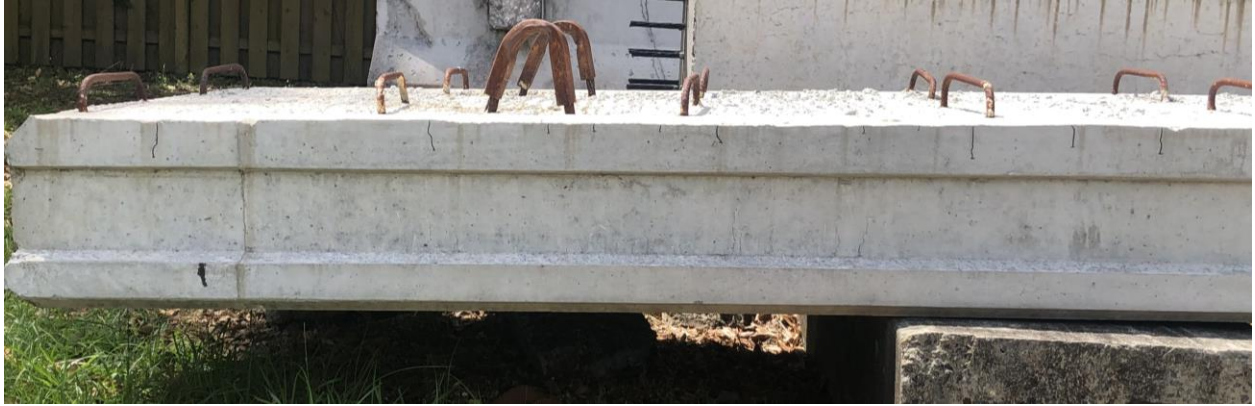
Figure 10 Cracks Noted at the End of the Slab
