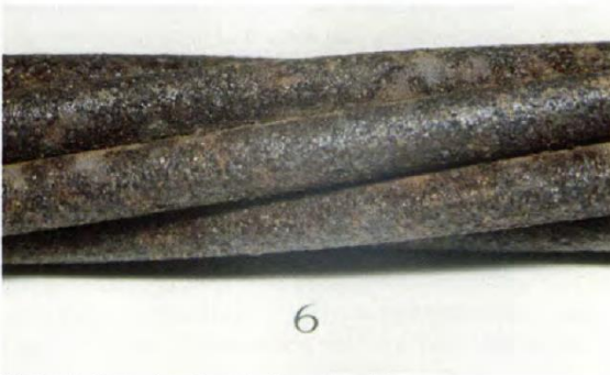
Photo 6. Strand surface before cleaning.
