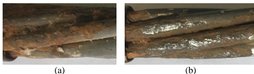
Figure 19-1. Corrosion rating = 6 for strand in 5 PC grout of 15 PC/5 PC D1C specimen: (a) Before cleaning; (b) After cleaning
