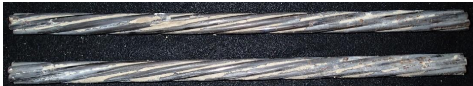
Figure 8-16. Corroded strands near port C control ISG specimen
