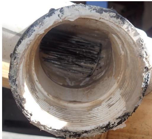
Figure 6-3. Soft grout removed at PVC tee inlet and outlet
