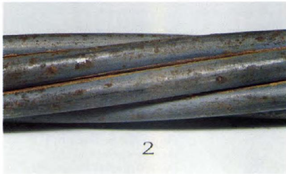
Photo 2. Strand surface before cleaning.
