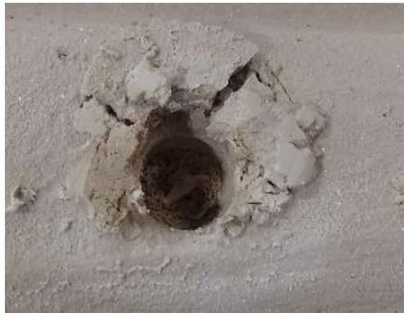
Figure 8-7. Soft grout as wet clayey sand
