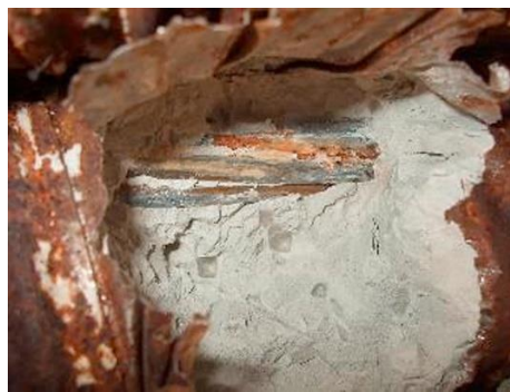
Figure 2-1. Deficient grout in PT (post-tensioned) tendon in Sicily, Italy (Anania et al., 2018)
