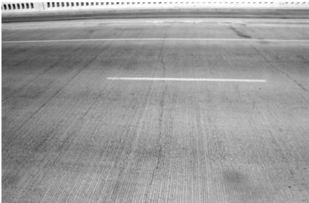
Figure 6: Transverse cracking (Frosch et al., 2003)
