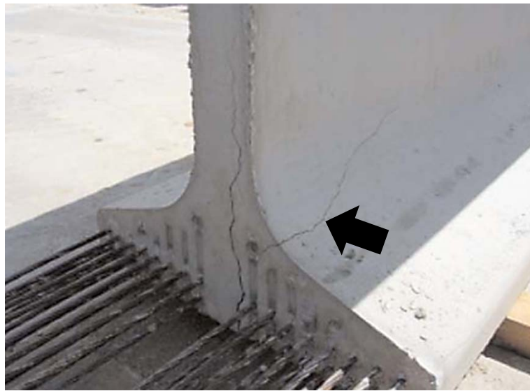
Figure 4—Flange splitting crack (Tadros et al. 2010)
