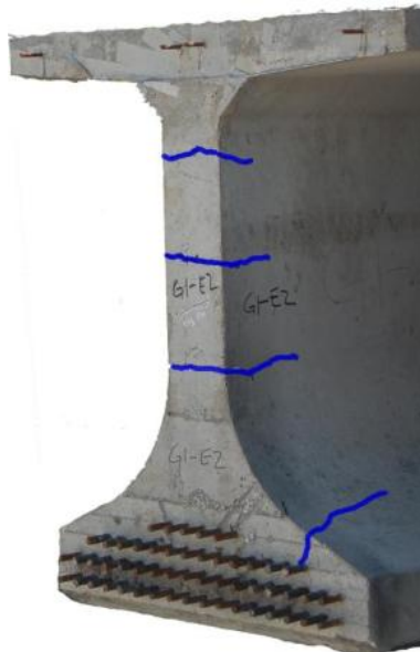
Figure 69–Web splitting and flange splitting cracks
