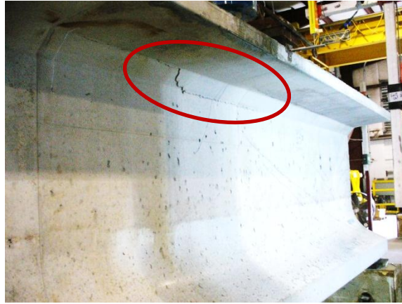
Figure 76–Punching shear failure in specimen SL
