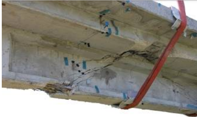
Figure 16–X7 punching failure bottom view
