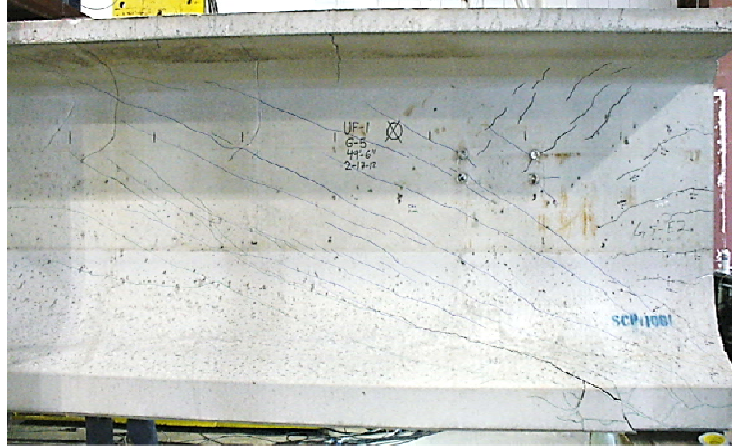
Figure 72–Bond shear failure of specimen SL
