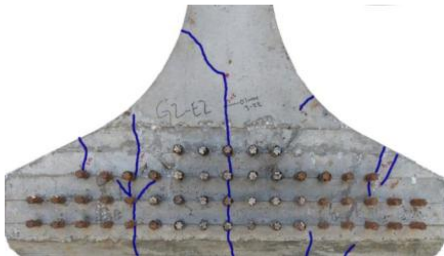
Figure 13–Flange splitting in experimental girder.
