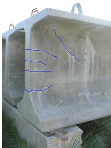
Figure 18–Web splitting cracks (enhanced in blue)
