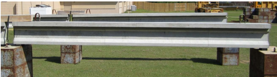
Figure 3-7: Picture of half-scale girder with cut strands and concrete repair
