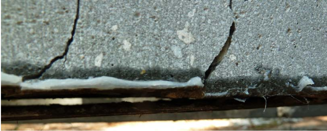
Figure 4-23: Close-up of laminate debonding initiated by flexural crack development
