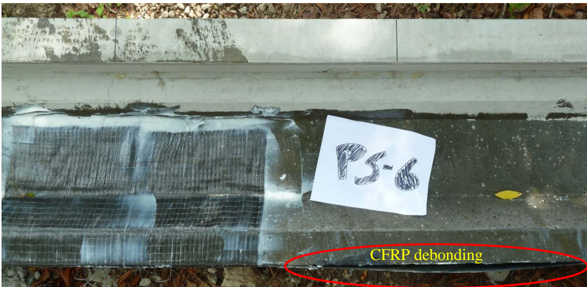
Figure 4-22: Half-scale girder displaying debonding failure of CFRP laminates
