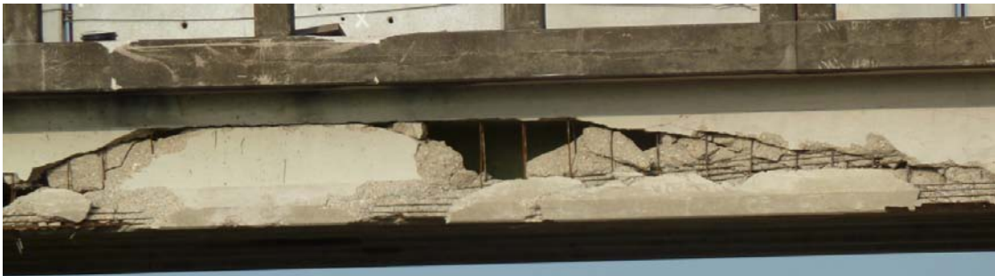
Figure 1-1: Example of severe impact damage to prestressed concrete bridge girder
