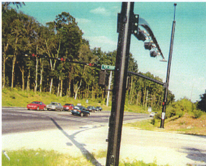
Figure 1.3: A Typical Lighting Installation in Service
