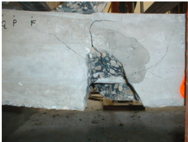
Figure 4.3 – Edge failure of Specimen B
